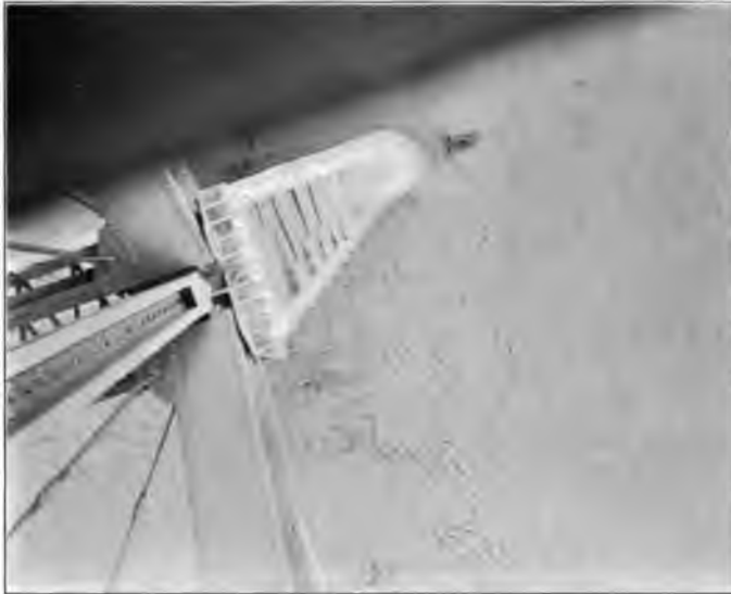
FIG. 1.—SMITH AVE. VIADUCT. VIEW LOOKING VERTICALLY DOWN AT EXPANSION AND FIXED SHOES OF 250-FT. SPANS ON ROCKER BENT, SHOWING ABSENCE OF BOLT ON DOWN STREAM SIDE.
